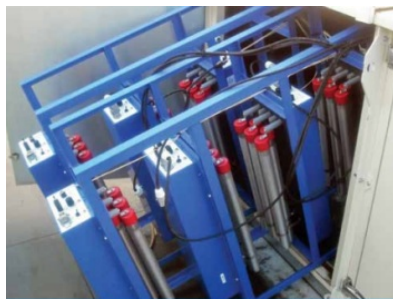
Racks of Ionizer Units
